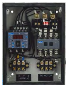
Interior View of MD Starter+ DOL Starter
